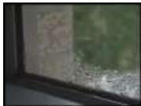
Condensation on windows
